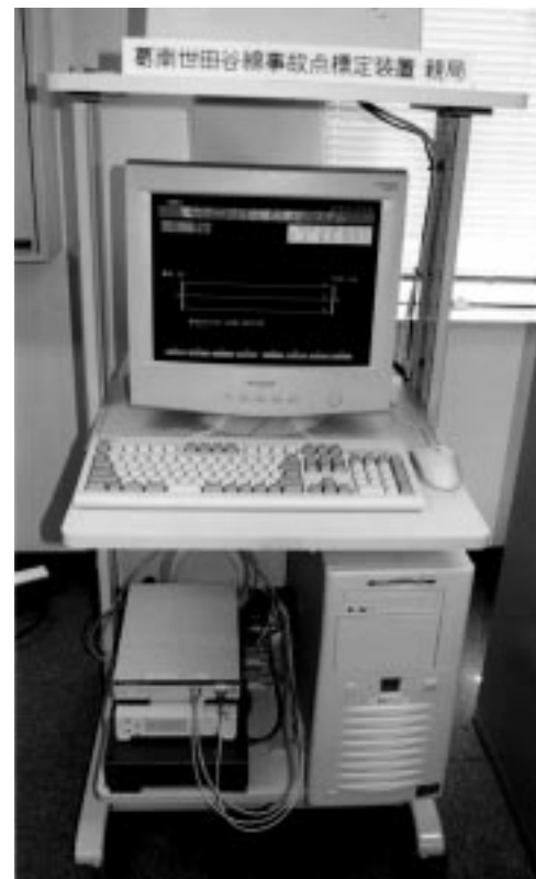
図7 親局外観 Appearance of master station
