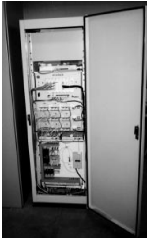
図5 子局外観 Appearance of local station
