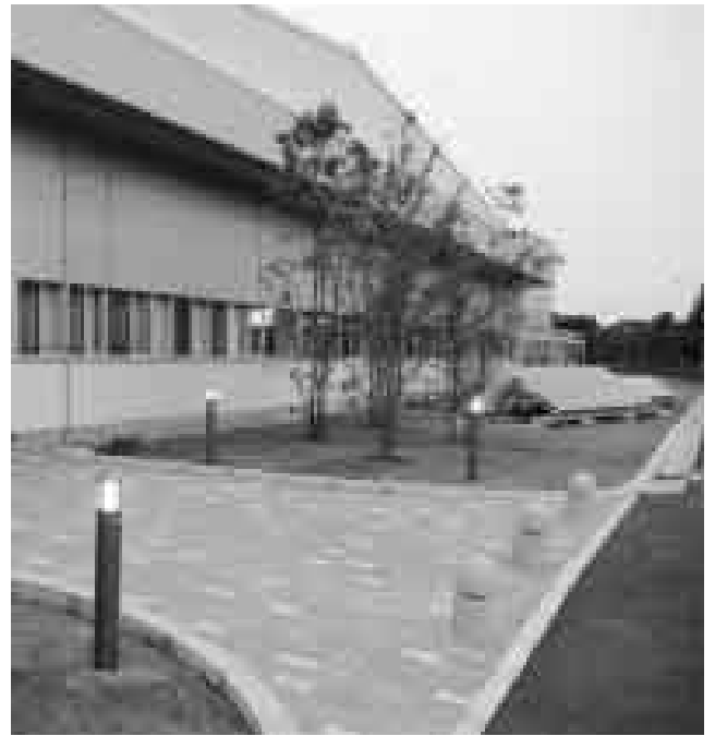
a) 誘導灯 a) Guide lights in outdoor.
