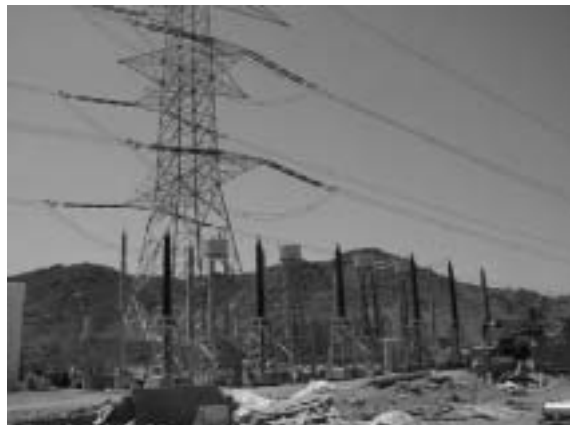
図5 新設分岐鉄塔と気中終端接続部 New tee off tower and outdoor sealing ends
