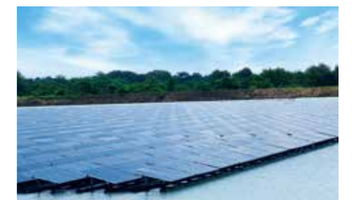
Floating solar panel installed in the reservoir inside FETL's Kabin Buri plant
