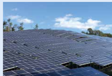
Example of construction: One of the largest solar farms in Japan Began operation in December 2019
