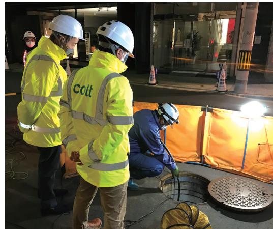
Mr. Hoshino, President and Head of Asia (pictured at left) of Colt Technology Services Co., Ltd. visiting the installation site for 3000-fiber WTC®
