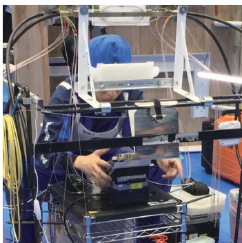
Splicing with Fujikura fusion splicer
